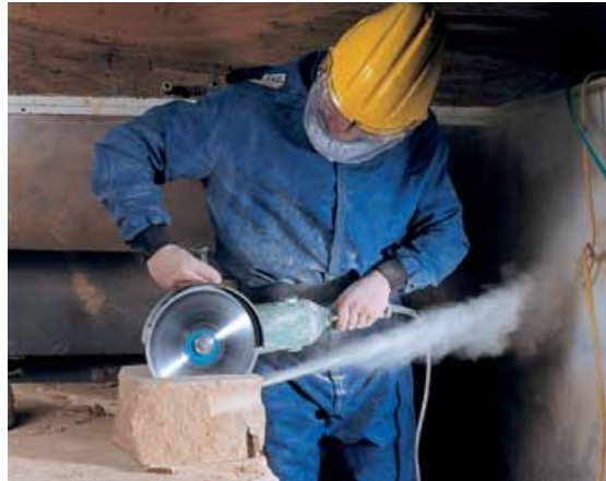
Photograph 3 Disc cutting control. Disc cutting in an exhaust ventilation booth – good dust control but poor working position. It would be better to have 'banker' on RHS and work side-on to the booth airflow
