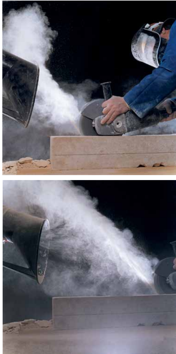
Photograph 10 Disc cutting using a captor hood. Stonemason attempting to direct dust jet into a captor hood with limited success at the start of the cut and almost no effective control at the end of the cut. Captor hoods cannot cope with large, fast moving dust-laden air jets.
